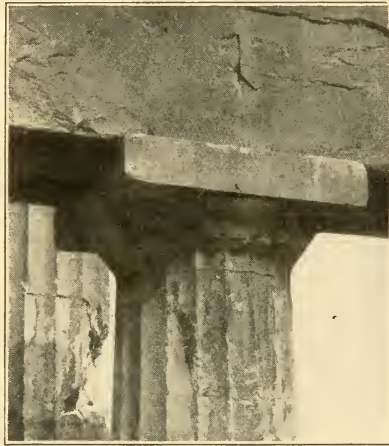
A DORIC CAPITAL. — From a photograph of a detail of the Parthenon (p. 107).
